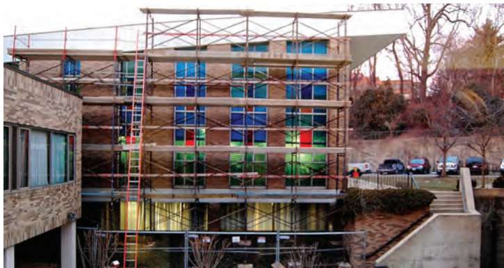
BEFORE: It was exciting to see the scaffold go up as Phase I – the renovation of our chapel – began.
