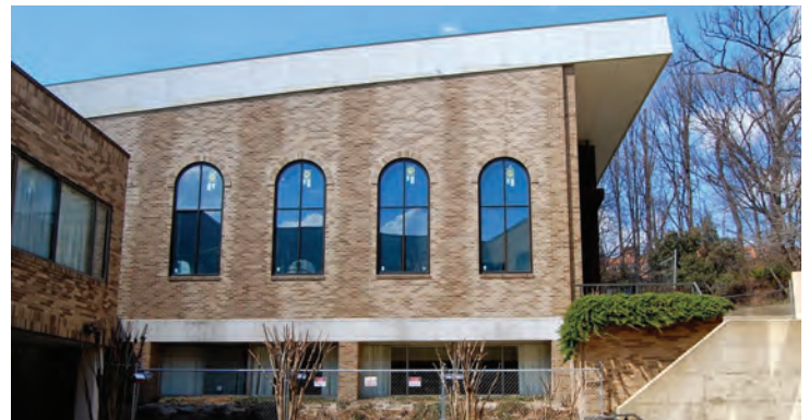
AFTER: It wasn't long before the single paned and leaky-windows were removed, brickwork repaired and double-paned energy efficient windows installed.
